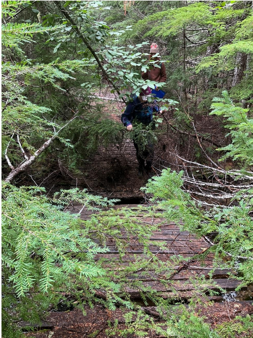
Old wooden foot bridge in disrepair
