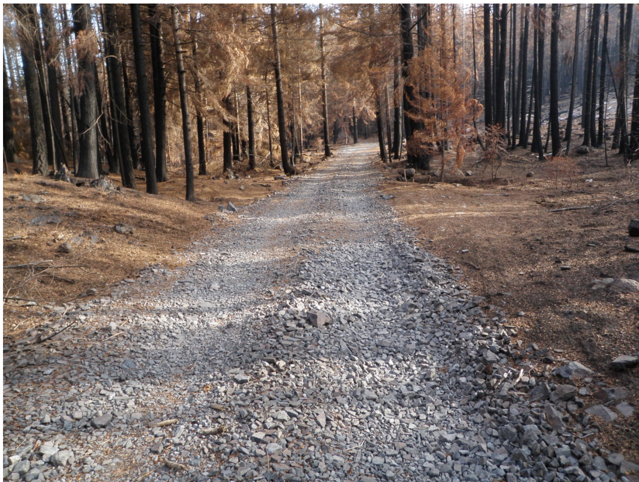
Figure 3-17: Photo showing the 1711 road crossing of an intermittent stream that is tributary to Mosier Creek. This crossing and the crossing shown in Figure 3-15 are the only Riparian Reserve stream crossings in moderate to high severity burn areas. This crossing is also flat and well rocked.
