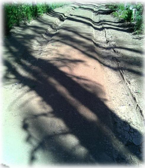
Figure 14220-130 Road contains little to no gravel and deep ruts.
