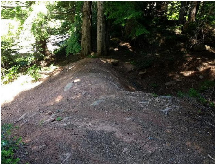
Ineffective closure at FSR 4610-040
