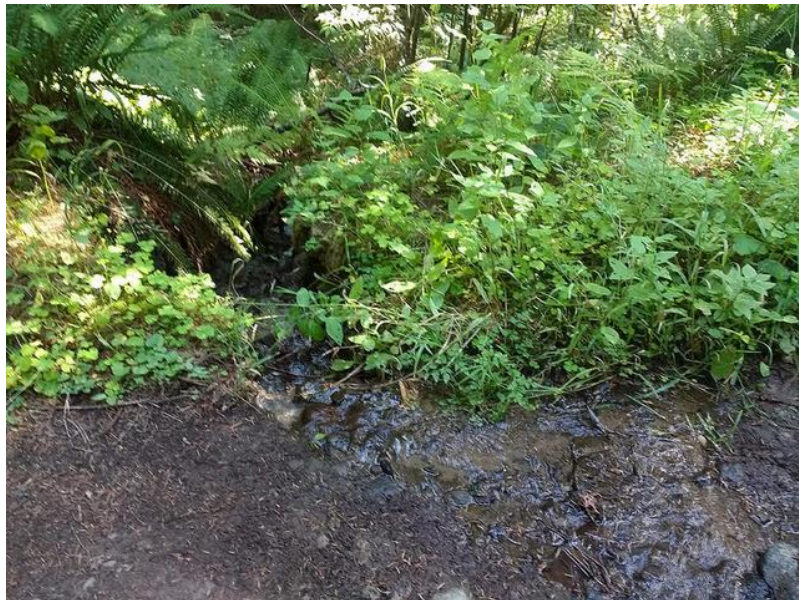
FSR 4614-120 crossing with Whisky Creek tributary – water seen flowing over roadbed and back into stream channel
